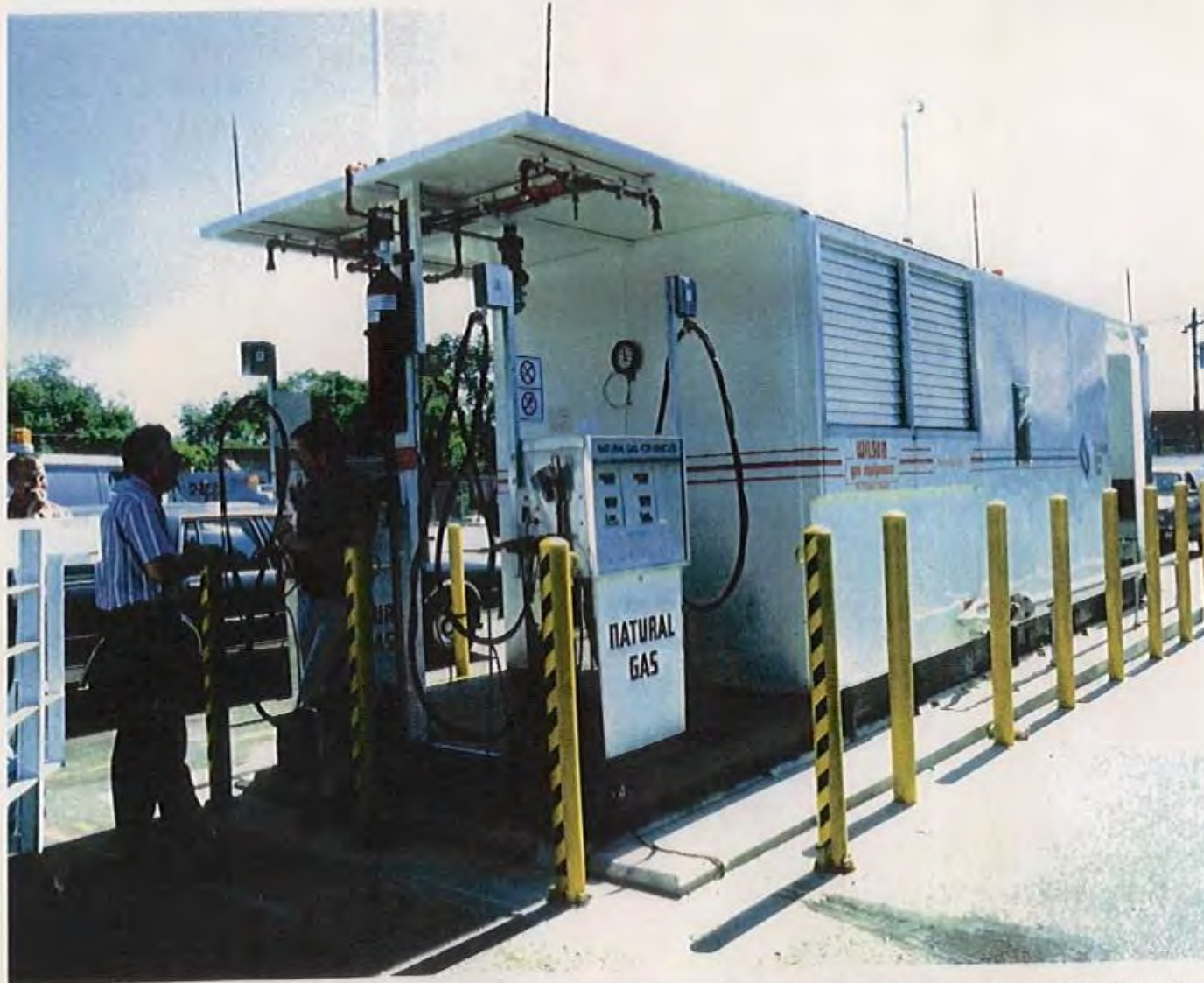
OGAS UNIT AND DISPENSERS SUPPLIED BY NUOVO PIGNONE TO BROOKLYN UNION GAS FOR DEDICATED CNG STATION IN NEW YORK
